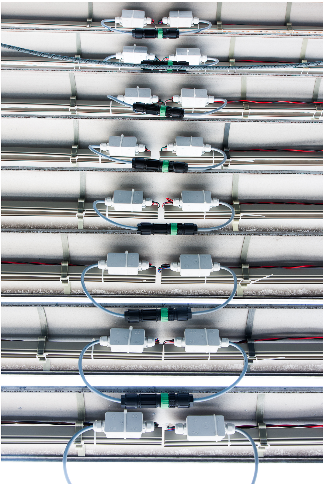
Figure 3.1: LED strips installed inside the sun blades of the computer science building.
