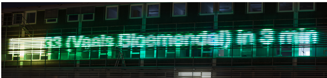
Figure C.2: Two columns with LED strips are still missing and one row on the left side is not working.
